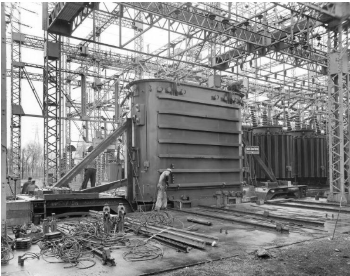
Dresser Power Station New Transformer, 1945 (Martin Collection, Indiana Historical Society)
