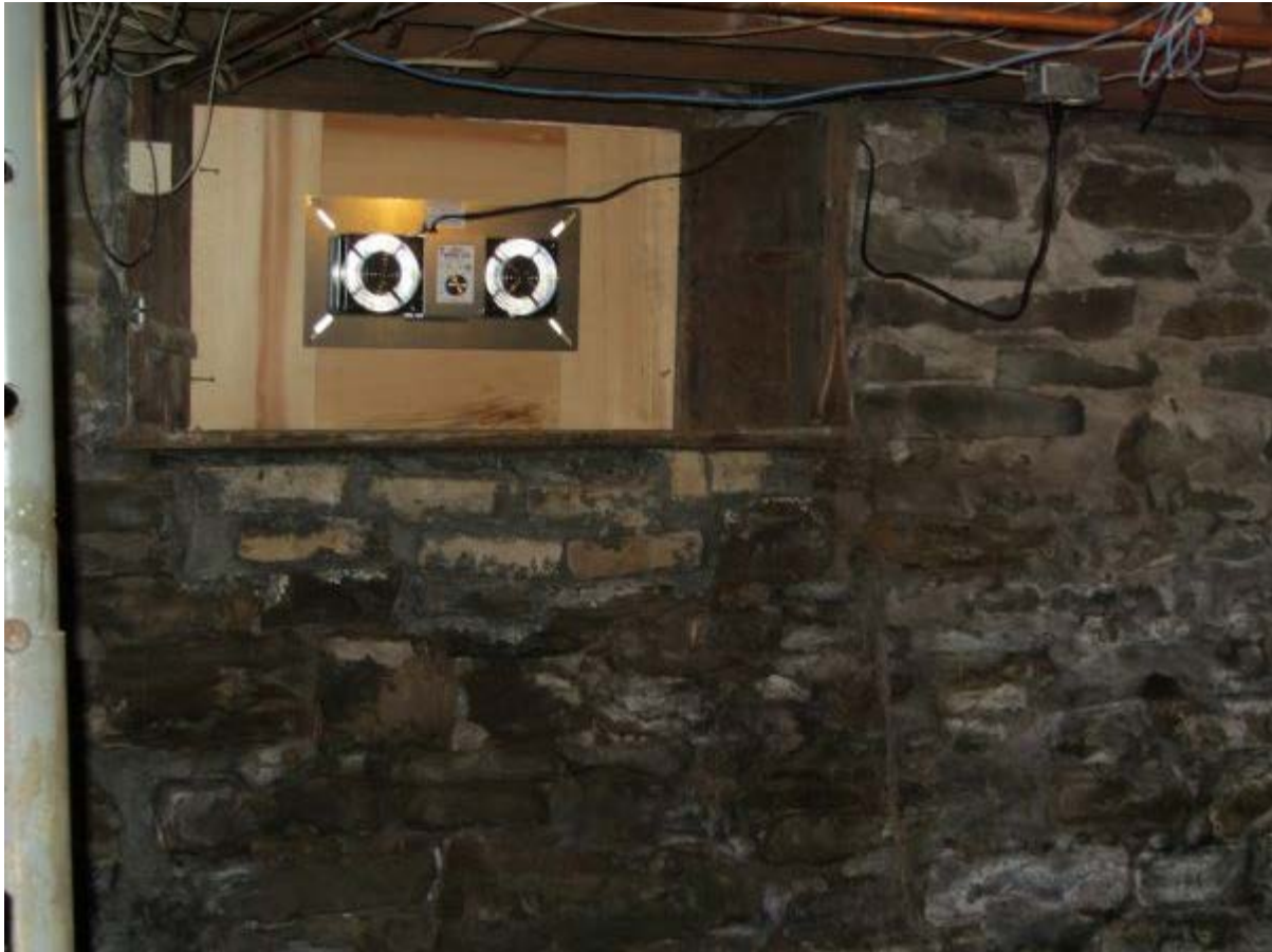
Ventilation fan controlled by a dehumidistat. (Image provided by Amanada Manahan)
