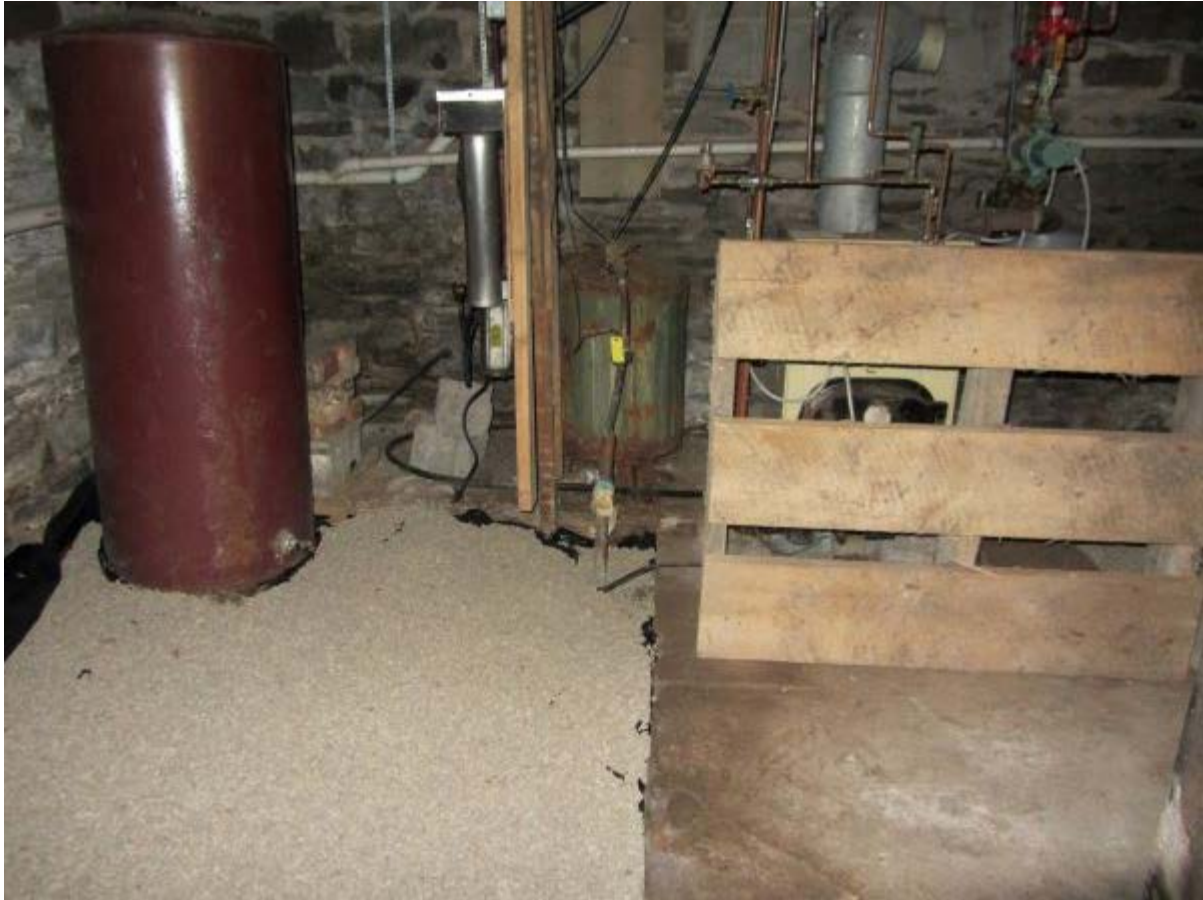
Dirt Floor covered with 6 mil of gravel. (Image provided by Amanda Manahan)
