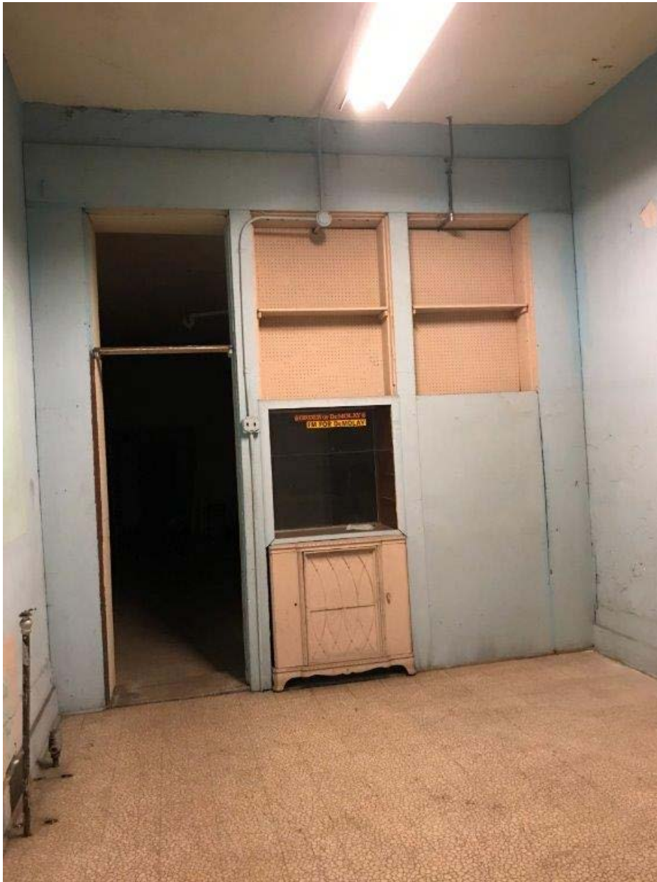
DeMolay Room, before. View looking north standing in the entrance doorway. The wall dividing the space was removed to create more flexibility.
