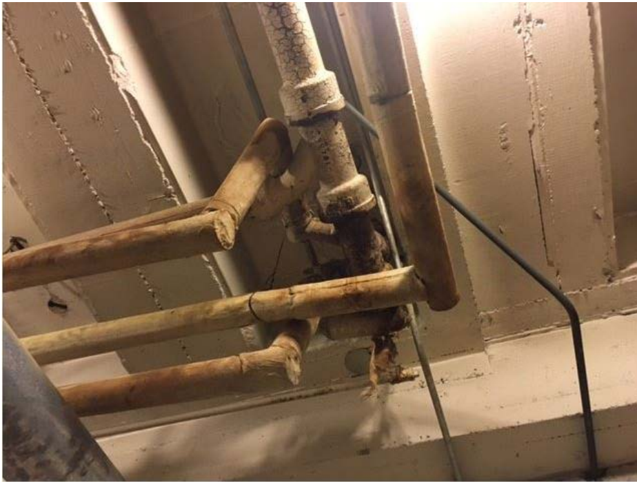
Pictured here are some of the pipes above one of our storage rooms. A piece of insulation had detached from the wrapping and was hanging above a storage shelf.
