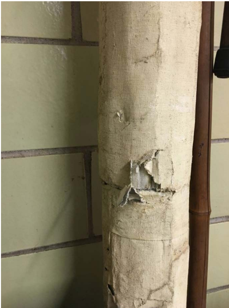
Crumbling asbestos wrapping found on a pipe at the museum.
