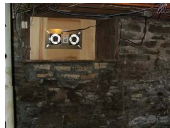
A ventilation fan controlled by a dehumidistat has been installed in this basement window to provide additional ventilation.
