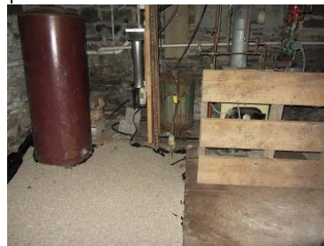
The dirt floor in this basement has been covered with 6 mil and a thin layer of gravel.
